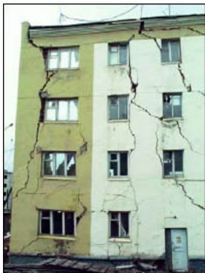
Cracking due to permafrost melting
